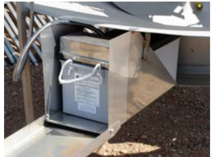
Battery Lid Down, Battery Lead Out
